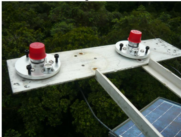
Paired Pyranometers (with protective caps used during installation)
