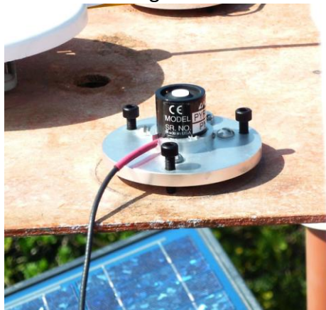
Close-up of Pyranometer
